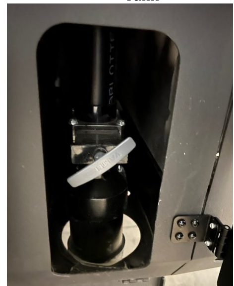
Figure 9-15: Grey Water Gate Valve
