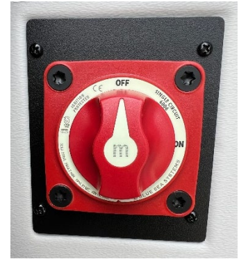
Figure 6-3: Battery Disconnect Switch
