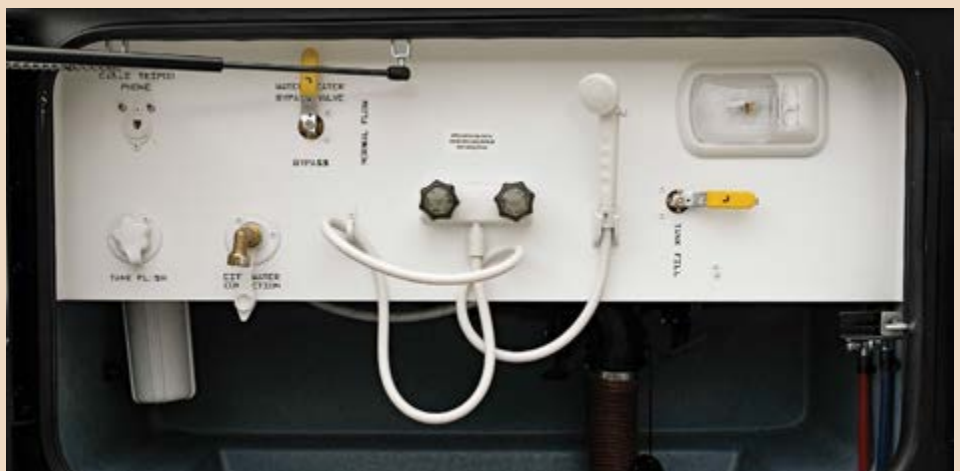
The lighted Tiffin utility bay conveniently locates the water filter, communications, tank flush, fresh water fill, outdoor shower for cleanup, water heater bypass, sewer connection, and low-point drain lines in one place. The 50-amp power supply is in a DS rear compartment.
