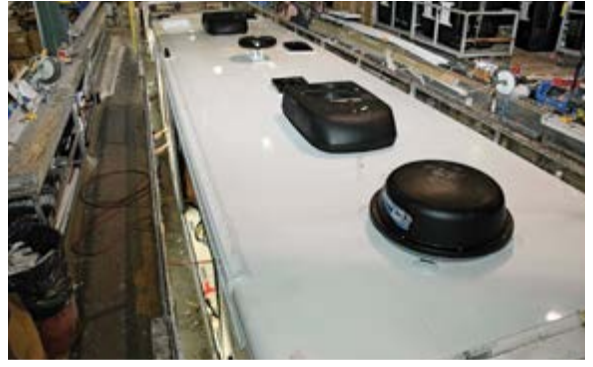
At Station 8, air conditioners, satellite receiver, TV antenna, and power vents are installed.
