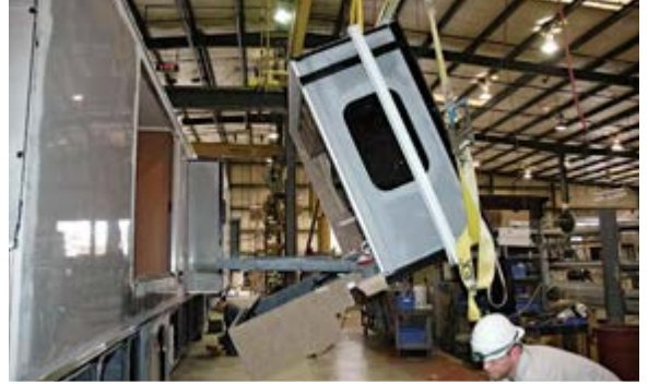
At Station 9, the slide-out for the bed is suspended from a sling while workmen move it into the wall opening. The heavier front slides are installed with power lifts.
