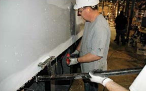
Operating as a team, one person aligns the wall with a leverage bar while another drives the 4-inch screws into the frame.
