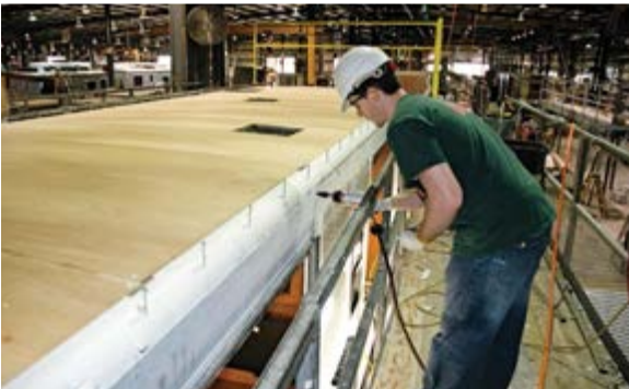
The fiberglass wall is attached to the side of the roof frame. Then screws are driven vertically through the roof assembly into the top of the wall assembly.
