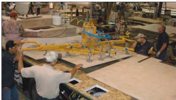
Pre-assembled ceramic tile or simulated hardwood floors are choices when the motorhome is custom-ordered. A vacuum crane lowers the assembly perfectly into place at Station 3.
