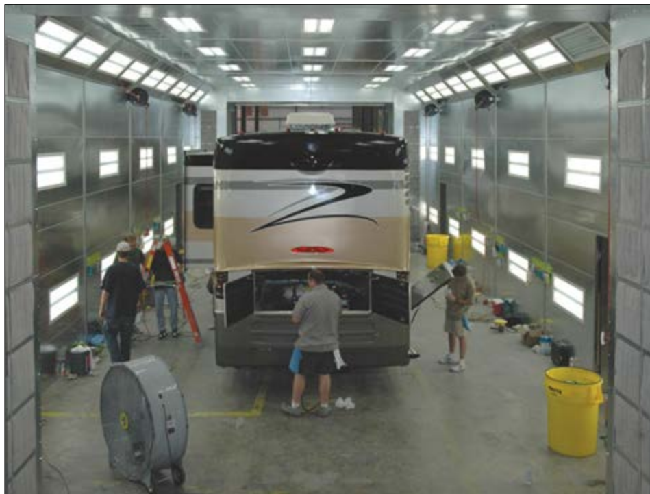
Global Finishing Systems of Carrollton, Texas, built 15 state-of-the-art paint booths with downdraft air control systems and finished the project three weeks early in May 2004.
