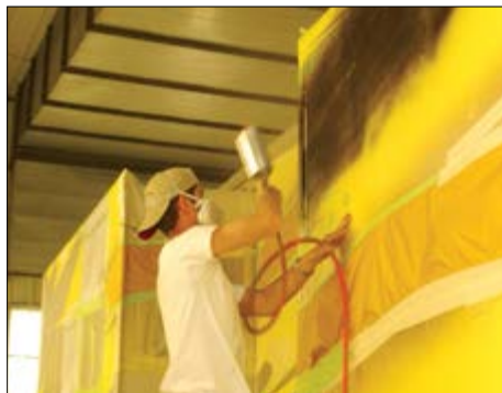
After one of the stripes has been painted in one of the three accent colors, Brian Murray covers the painted area with a paper mask to protect the paint as the next accent color is applied by John Gordon.
