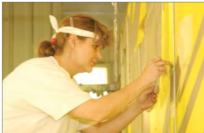
With the base coat of paint completed and dry, Robert Borden, Randy Page, and Craig Rogers align the first roll of striping masks over the storage bay doors and wheel wells of an Allegro Bay. After the adhesive backing is carefully removed, Randy Page presses the air bubbles out of the mask with an edging tool. Renae Scott does the detail work in fitting the mask over molding.
