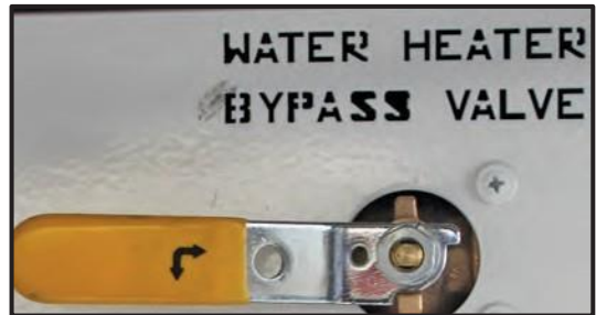
Figure 0-9: Water Heater Bypass System
