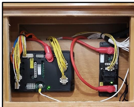
Figure 0-3: Multiplex System Switch Panel
