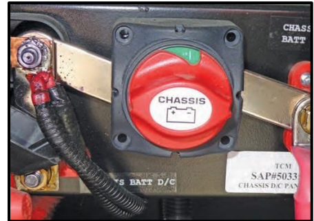
Figure 0-16: Engine Battery Disconnect Switch
