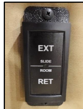
Figure 0-2: Front Slide-Out Switch
