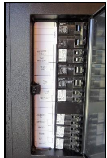
Figure 0-4: Circuit Breaker Boxes
