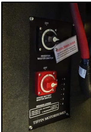
Figure 0-15: House Battery Disconnect Panel
