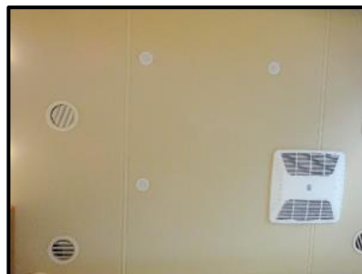
Figure 0-3: Supply Vents and A/C Unit
