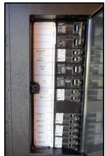
Figure 0-4: Circuit Breaker Boxes
