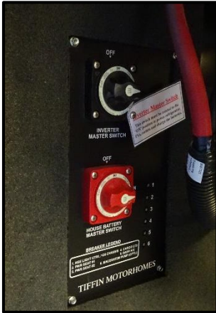
Figure 0-15: House Battery Disconnect Panel
