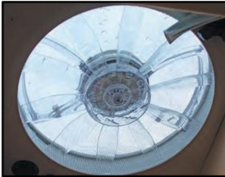
Figure 0-3: Overhead Vent Fan
