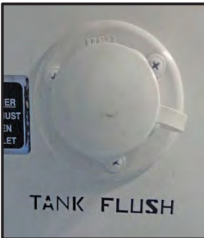
Figure 13-13: Tank Flush Connection
