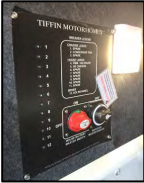
Figure 9-17: House Battery Disconnect Panel
