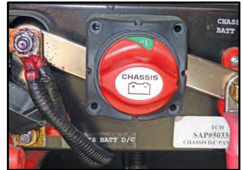
Figure 9-18 Engine Battery Disconnect Switch. Front Wall of Battery Camp
