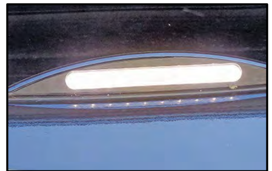
Figure 11-3: Exterior Security Light
