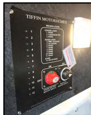
Figure 9-13: 12 VDC Breaker Buttons
