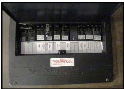
Figure 9-5: 120 VAC Circuit Breaker Box
