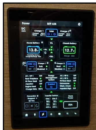
Figure 8-13: Control Panel for the Inverter/Charger
