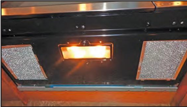
Figure 4-3: Air Filtration Fan
