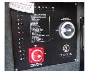
Figure 8-4: House Battery Disconnect Panel Switch
