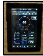
Figure 3-6: Heat Pump Controls
