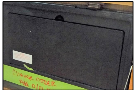
Figure 8-1: Circuit Breaker Box
