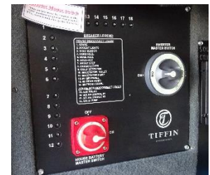
Figure 8-4: House Battery Disconnect Panel Switch
