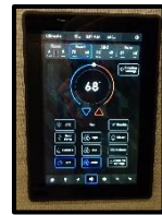
Figure 3-6: Heat Pump Controls
