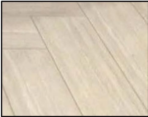
Figure 11-2: Typical Flooring in the Zephyr
