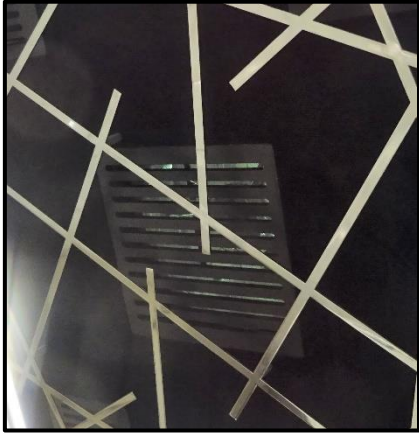
Figure 13-6: Overhead Vent Fan
