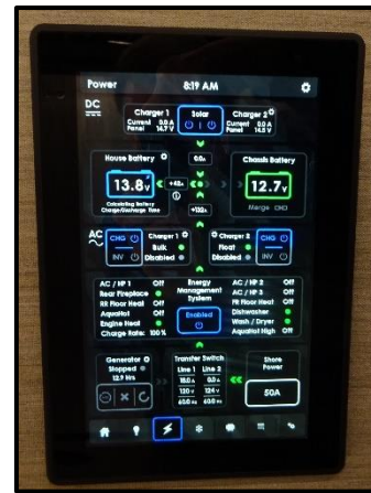
Figure 8-13: Control Panel for the Inverter/Charger
