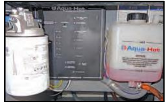
Figure 12-16: Aqua-Hot Surge Tank
