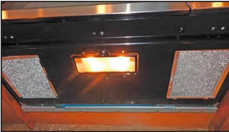
Figure 4-3: Air Filtration Fan
