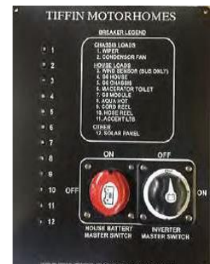
Figure 8-5: House Battery Disconnect Panel Switch
