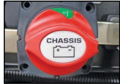
Figure 8-6: Engine Battery Disconnect Panel Switch
