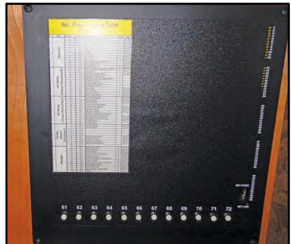
Figure 8-1: Circuit Breaker Box
