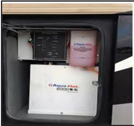
Figure 3-2: Aqua-Hot Surge Tank
