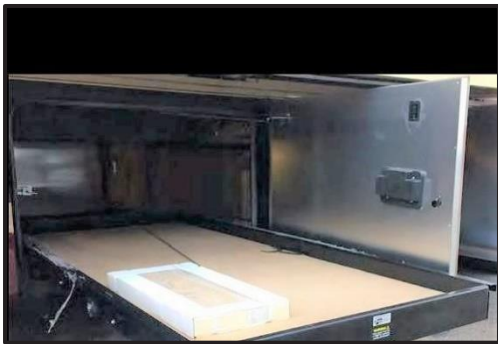
Figure 8-4: House Battery Disconnect Switch Location *** confirm image for Zephyr ***
