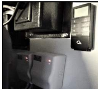
Figure 13-5: Awning Remote Control Module (located in the cargo bay)
