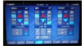
Figure 3-7: Heat Pump Controls
