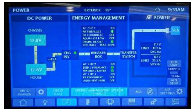
Figure 8-12: Control Panel for the Inverter/Charger
