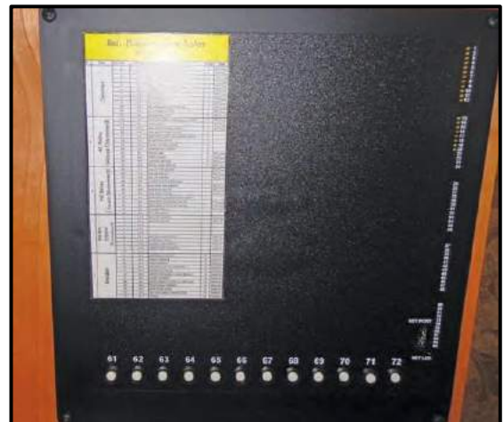
Figure 8-1: Circuit Breaker Box
