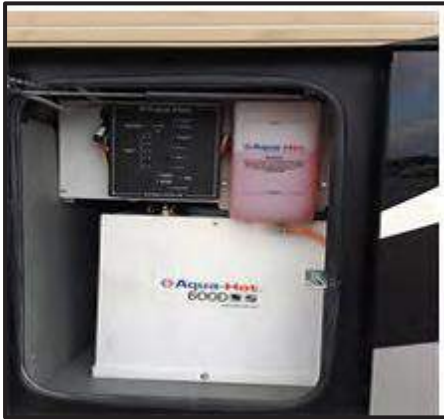
Figure 3-2: Aqua-Hot Surge Tank
