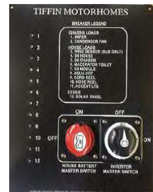
Figure 8-5: House Battery Disconnect Panel Switch
