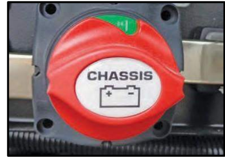
Figure 8-6: Engine Battery Disconnect Panel Switch
