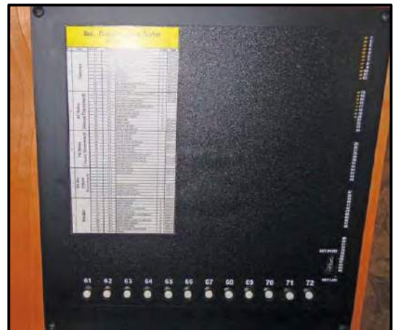
Figure 8-2: Circuit Breaker Box
