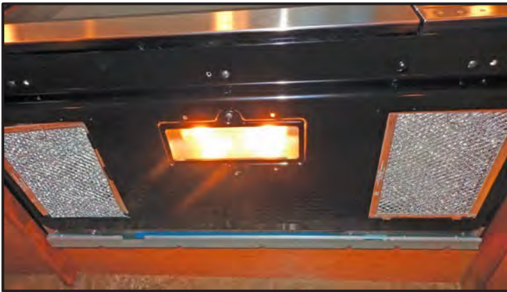
Figure 4-3: Air Filtration Fan
