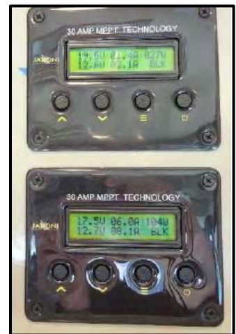
Figure 8-1: Solar Panel Controls
