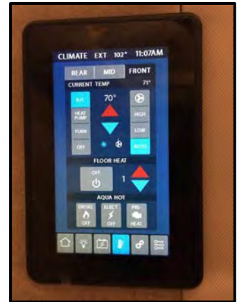
Figure 3-8: Heat Pump Controls
