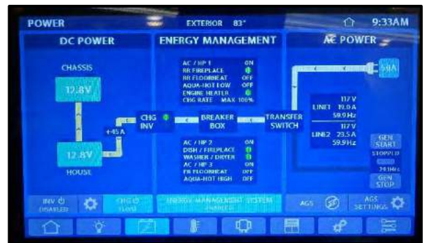
Figure 8-11: Control Panel for the Inverter/Charger
