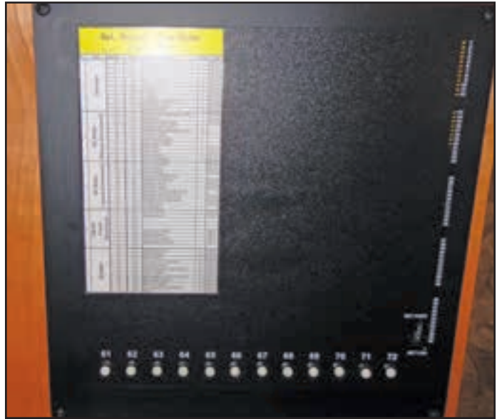
Figure 8-1: Circuit breaker box
