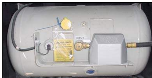
Figure 2-4. Liquid Propane Tank
