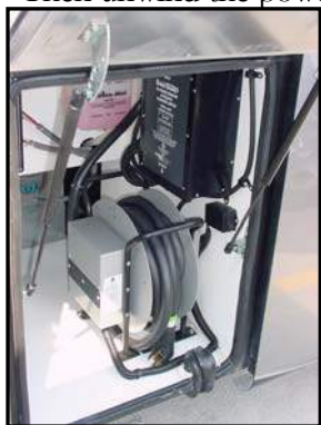
Figure 7-2. Electrical Power Hookup Cable
