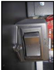
Figure 7-17. Power Switch for Generator
