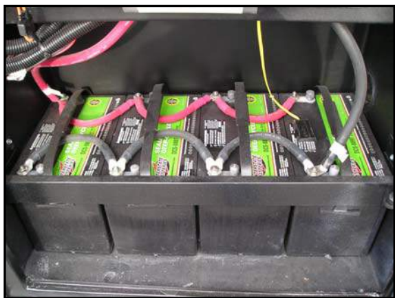
Figure 7-6. Maintenance Free House Batteries (Compartment)
