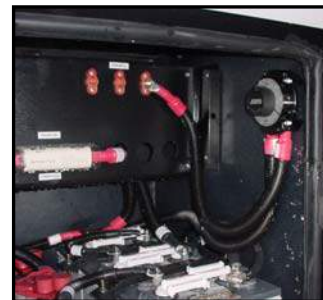
Figure 7-9. Rotary Switch to Disconnect “House” Batteries
