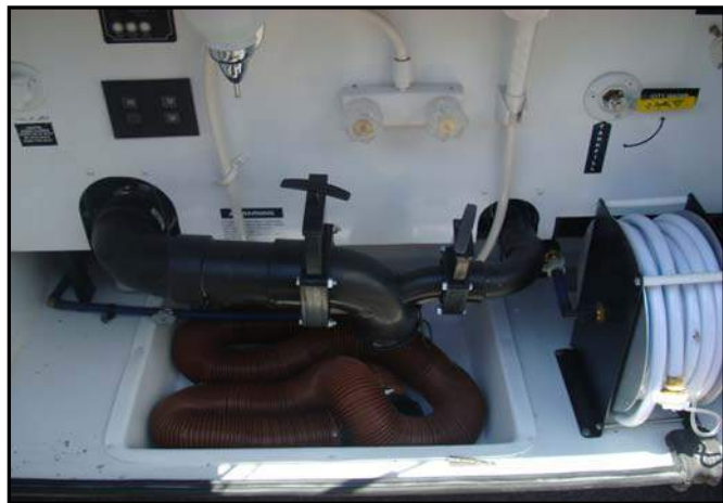
Figure 11-10. Sanitation Compartment Containing Holding Tank Drains and Flexible Drain Hose
