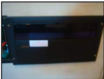
Figure 7-3. Circuit Breaker Box
