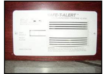
Figure 3-9. CO/LP Gas Detector
