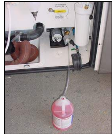
Figure 14-17. Winterizing the Water System
