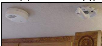
Figure 2-8. Smoke Detector (Left)
