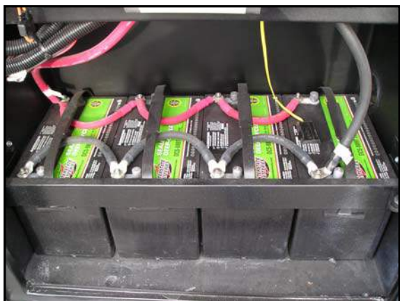
Figure 7-6. Maintenance Free House Batteries (Compartment)
