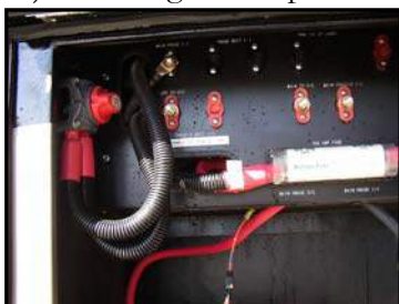
Figure 7-8. Rotary Switch to Disconnect Engine Battery
