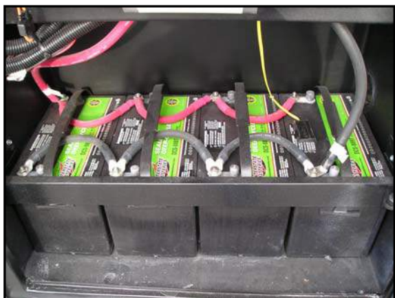
Figure 7-6. Maintenance Free House Batteries (Compartment)
