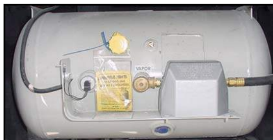
Figure 2-5. Liquid Propane Tank
