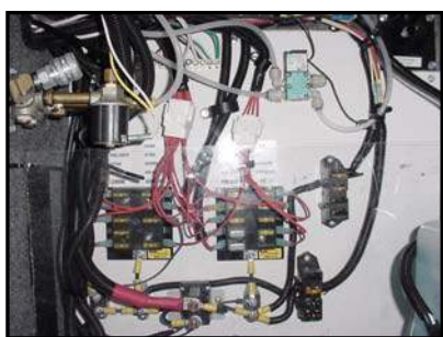
Figure 7-4. 12 VDC Fuse Panels
