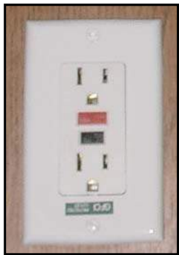
Figure 7-13. Ground-Fault Circuit Interrupter (GFCI)
