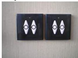
Figure 10-6. Control for Passenger & Entry Door Power Shades
