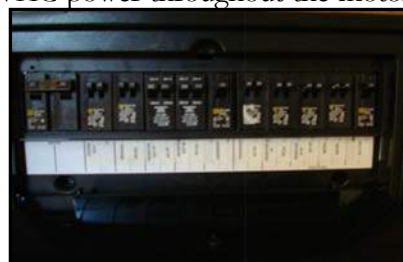
Figure 7-15. Energy Management System
