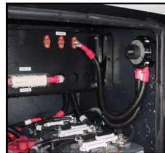
Figure 7-9. Rotary Switch to Disconnect “House” Batteries
