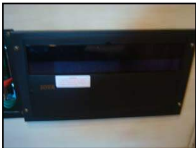
Figure 7-3. Circuit Breaker Box
