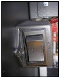
Figure 7-17. Power Switch for Generator
