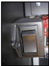
Figure 7-16. Power Switch for Generator
