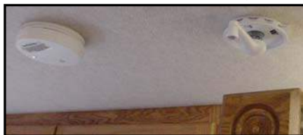
Figure 2-8. Smoke Detector (Left)
