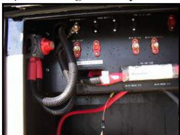
Figure 7-8. Rotary Switch to Disconnect Engine Battery
