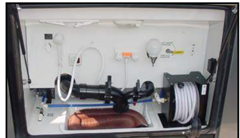
Figure 11-15. Exterior Shower in Outside Compartment
