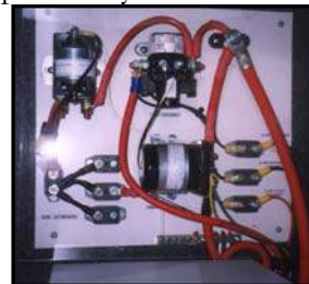
Figure 7-18. Resettable Circuit Breakers
