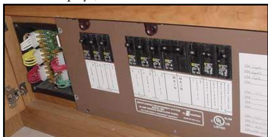
Figure 7-3. Circuit Breaker Box
