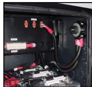
Figure 7-8. Rotary Switch to Disconnect “House” Batteries
