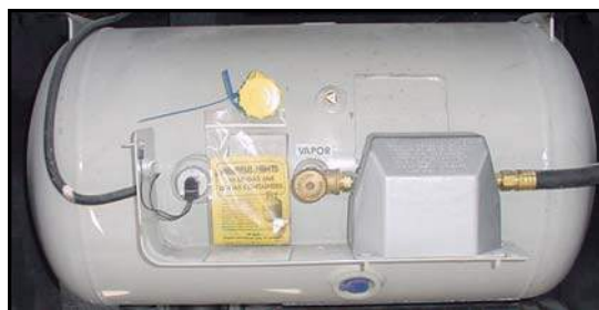
Figure 2-5. Liquid Propane Tank
