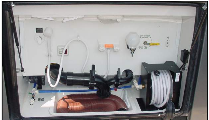
Figure 11-13. Sanitation Compartment Containing Holding Tank Drains and Flexible Drain Hose
