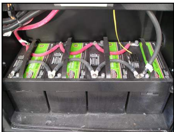
Figure 7-6. Maintenance Free House Batteries (Compartment)
