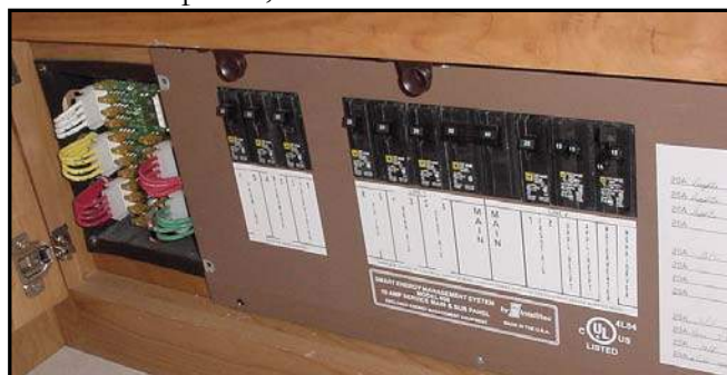
Figure 7-1. Circuit Breakers Located Under Refrigerator or in Bedroom Closet
