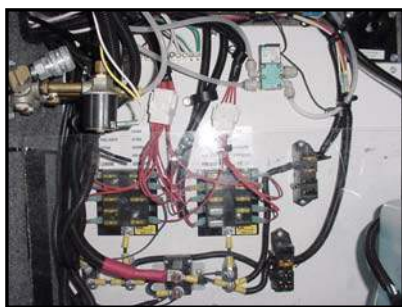
Figure 7-4. 12 VDC Fuse Panels
