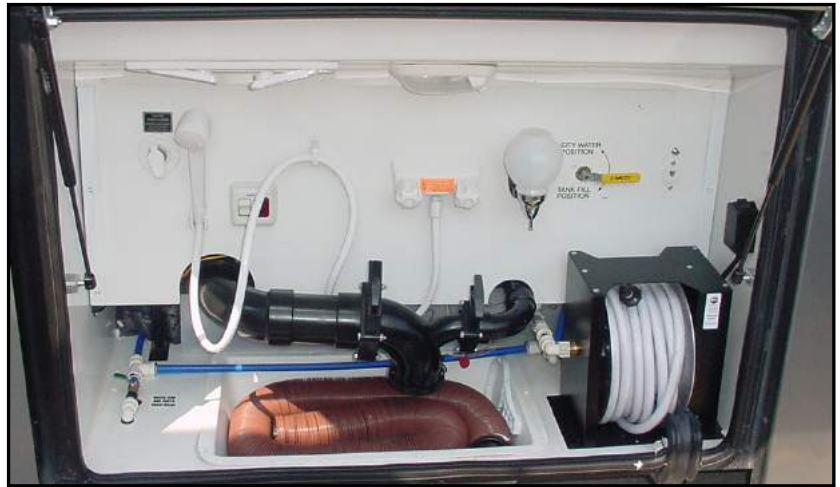
Figure 11-14. Sanitation Compartment Containing Holding Tank Drains and Flexible Drain Hose
