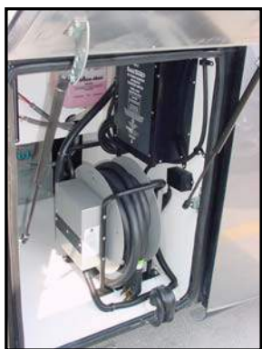
Figure 7-2. Electrical Power Hookup Cable
