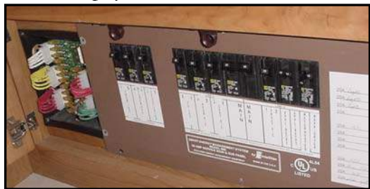
Figure 7-3. Circuit Breaker Box
