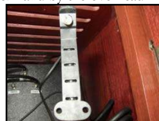
Figure 4-8. Stem inside cabinet
