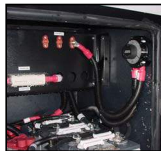
Figure 7-8. Rotary Switch to Disconnect “House” Batteries
