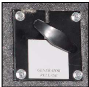
Figure 7-16. “Pull” Cable for Generator Release
