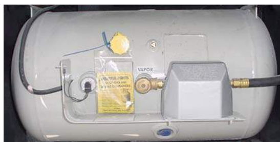
Figure 3-4. Liquid Propane Tank
