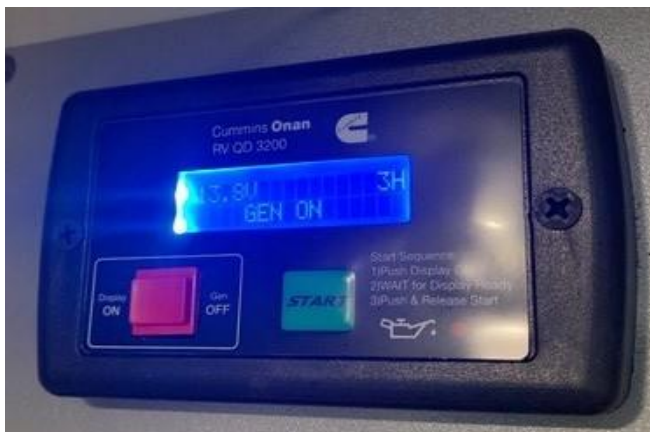
Figure 9-10: Central Control Panel
