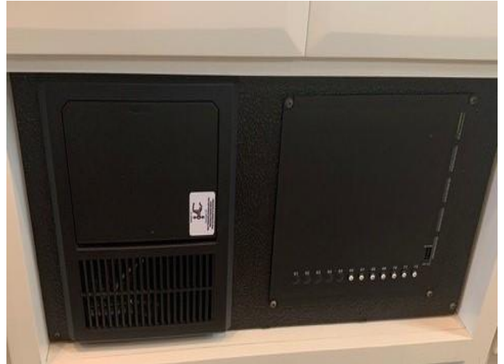
Figure 9-1 Electrical Breaker/Fuse Box
