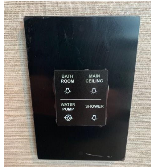
Figure 14-5: Water Pump Switches
