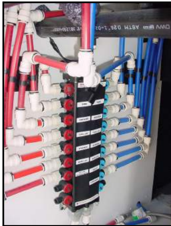
Figure 11-10. Water System Plumbing Manifold
