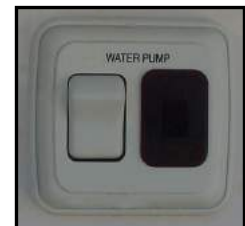
Figure 11-6. Water Pump Switch
