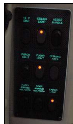
Figure 7-9. 12 VDC Disconnect Switch
