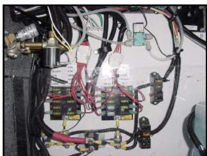
Figure 7-4. 12 VDC Fuse Panels
