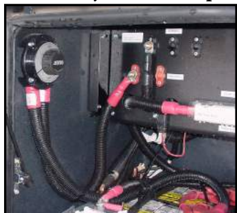
Figure 7-7. Rotary Switch to Disconnect Engine Battery
