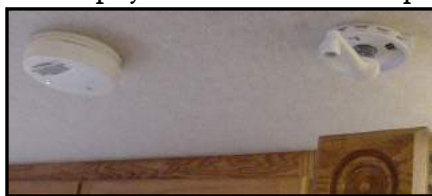
Figure 2-7. Smoke Detector (Left)
