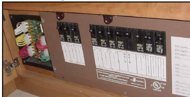
Figure 7-1. Circuit Breakers Located Under Refrigerator
