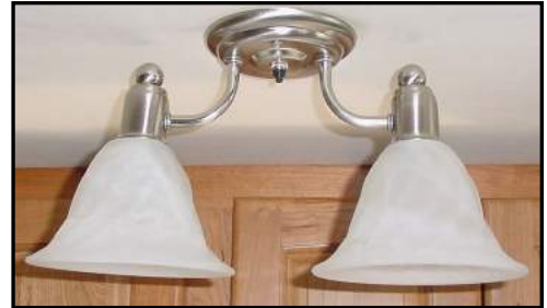
Figure 14-16. Typical Lighting Fixtures
