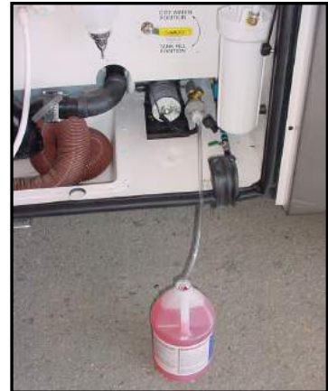
Figure 14-16. Winterizing the Water System
