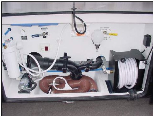
Figure 11-15. Sanitation Compartment Containing Holding Tank Drains and Flexible Drain Hose
