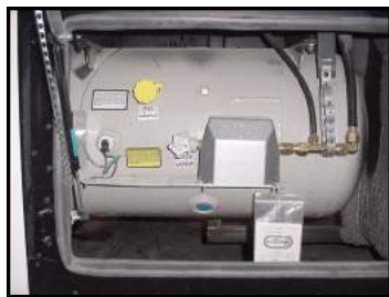
Figure 3-3. Liquid Propane Tank
