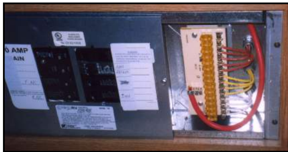
Figure 7-1. Circuit Breaker Box
