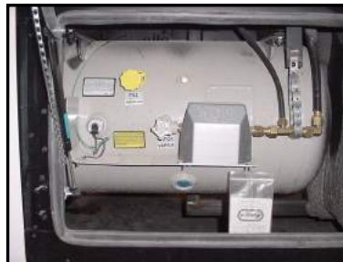
Figure 2-3. Liquid Propane Tank
