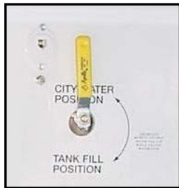
Figure 11-9. Water Fill Valve
