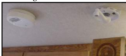
Figure 2-6. Smoke Detector (Left)
