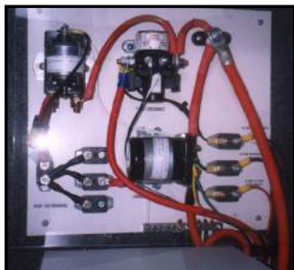
Figure 7-18. Resettable Circuit Breakers
