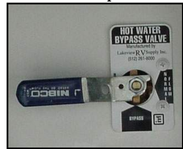
Figure 11-11. Water Heater Bypass
