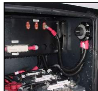
Figure 7-7. Rotary Switch to Disconnect "House" Batteries
