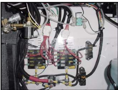
Figure 7-2. 12 VDC Fuse Panels
