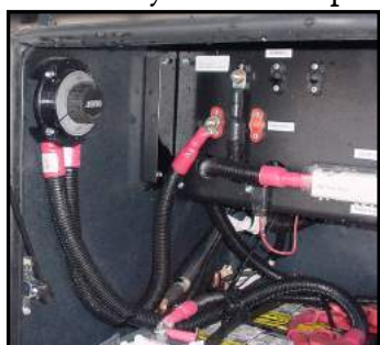
Figure 7-6. Rotary Switch to Disconnect Engine Battery
