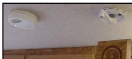
Figure 2-6. Smoke Detector (Left)
