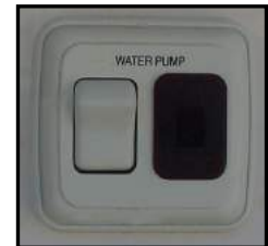
Figure 11-6. Water Pump Switch
