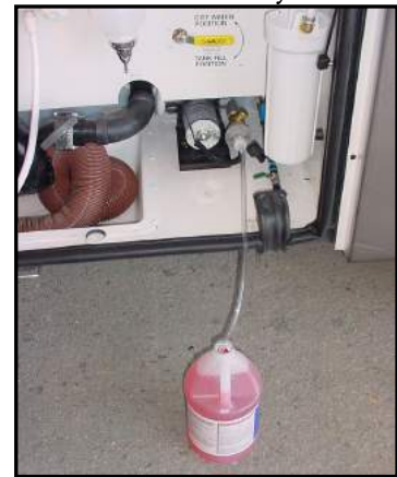
Figure 14-12. Winterizing the Water System
