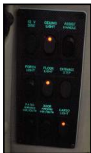
Figure 7-8. 12 VDC Disconnect Switch
