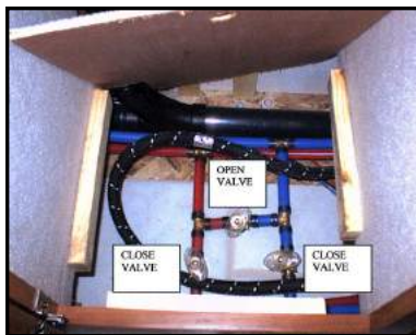
Figure 11-9. Water Heater Bypass
