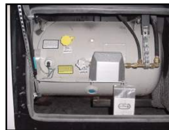
Figure 3-3. Liquid Propane Tank
