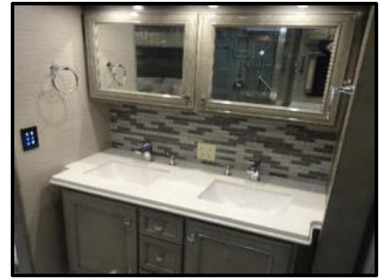
Figure 15-4: Bathroom Sink and Faucet
