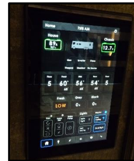
Figure 15-6: Spider Controls System Switch
