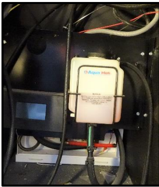
Figure 5-2: Aqua-Hot Surge Tank
