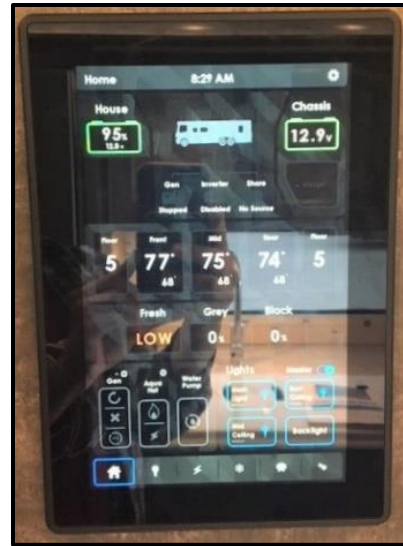
Figure 4-1: Home Screen for the Spyder Controls System
