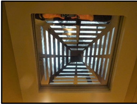
Figure 16-4: Overhead Vent Fan
