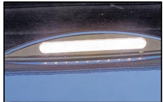
Figure 12-2: Exterior Security Light
