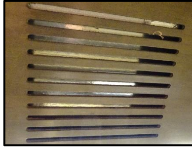
Figure 4-5: Return Air Vent
