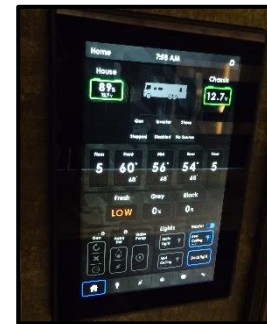
Figure 14-6: Spider Controls System Switch
