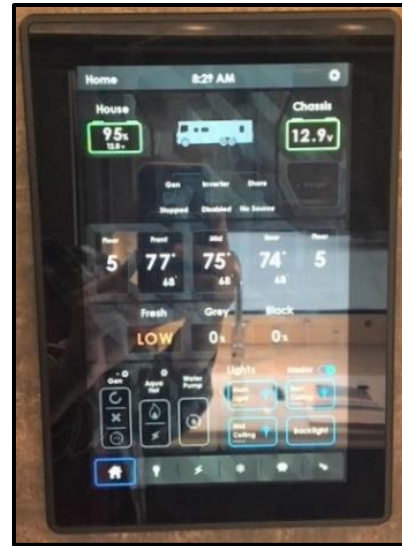
Figure 3-1: Home Screen for the Spyder Controls System
