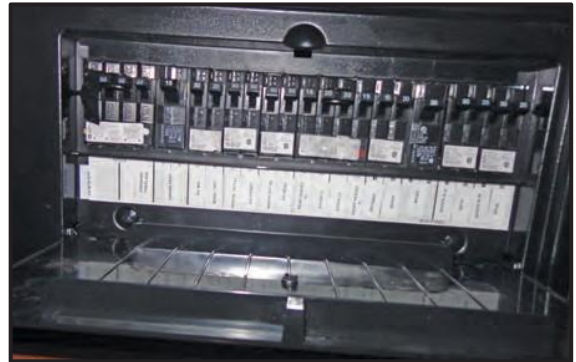
Figure 10-1: Circuit Breaker Boxes
