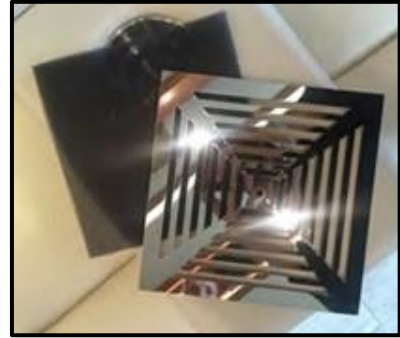
Figure 4-6: Air Vent Filter
