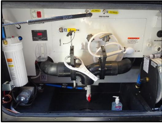
Figure 14-2: Location of Tank-Level Monitor in Plumbing Panel
