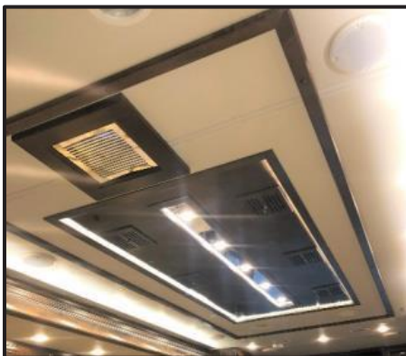
Figure 13-5: Typical Ceiling in the Phaeton
