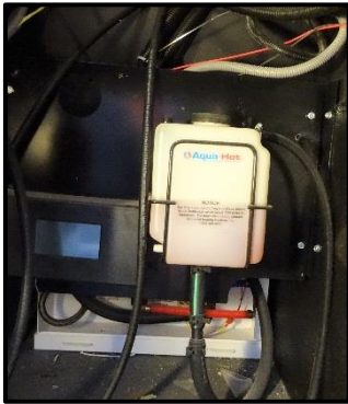
Figure 4-2: Aqua-Hot Surge Tank
