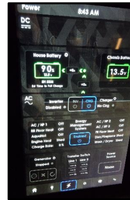
Figure 10-13: Energy Management System
