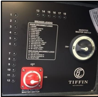
Figure 10-4: House Battery Disconnect Panel
