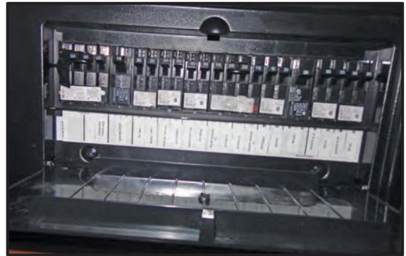
Figure 10-1: Circuit Breaker Boxes
