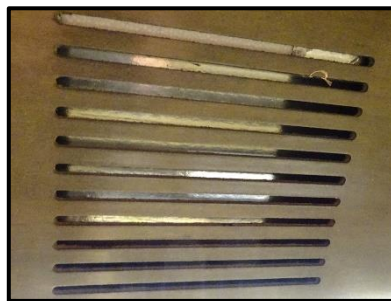
Figure 4-5: Return Air Vent
