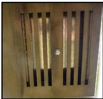
Figure 4-4: Outgoing Air Vent
