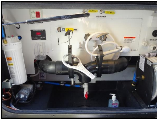
Figure 14-2: Location of Tank-Level Monitor in Plumbing Panel
