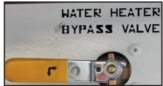
Figure 14-10: Water Heater Bypass System
