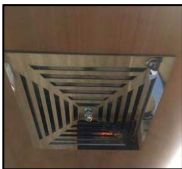
Figure 4-4: Outgoing Air Vent
