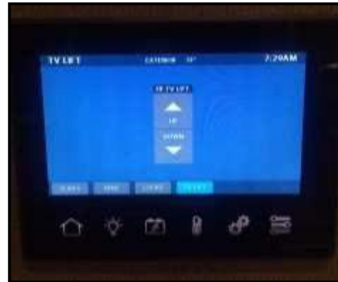
Figure 7-6: Spyder Controls System Panel
