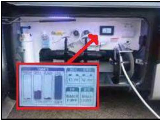
Figure 14-2: Location of Tank-Level Monitor in Plumbing Panel
