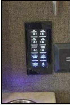
Figure 7-7: Television Lift Control Panel (located in the living room slide-out box)
