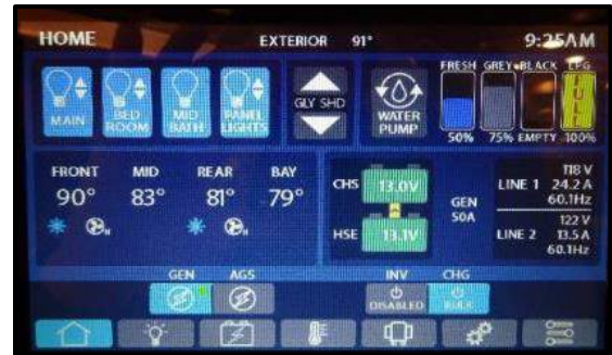
Figure 3-1: Home Screen for the Spyder Controls System
