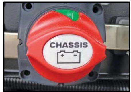
Figure 10-6: Engine Battery Disconnect Switch
