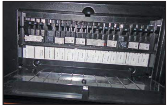
Figure 10-1: Circuit Breaker Boxes
