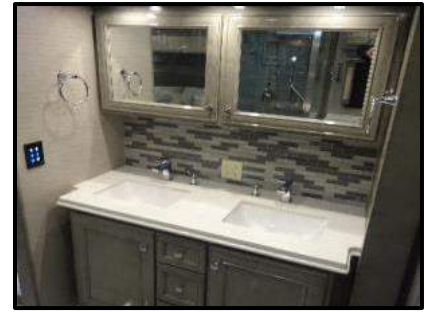
Figure 14-4: Bathroom Sink and Faucet
