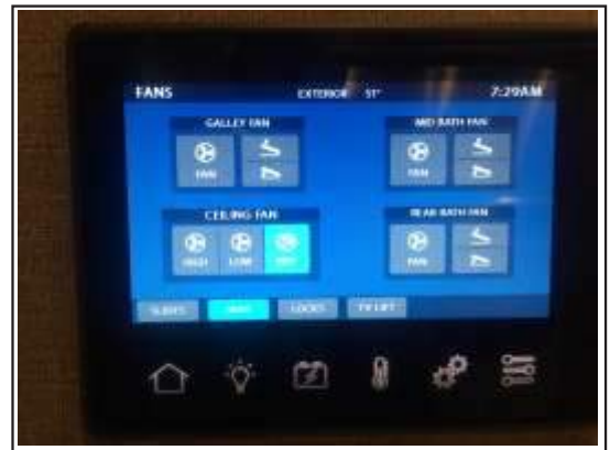
Figure 15-5: Vent and Fan Controller
