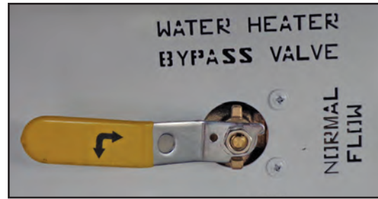
Figure 14-8: Water heater bypass valve
