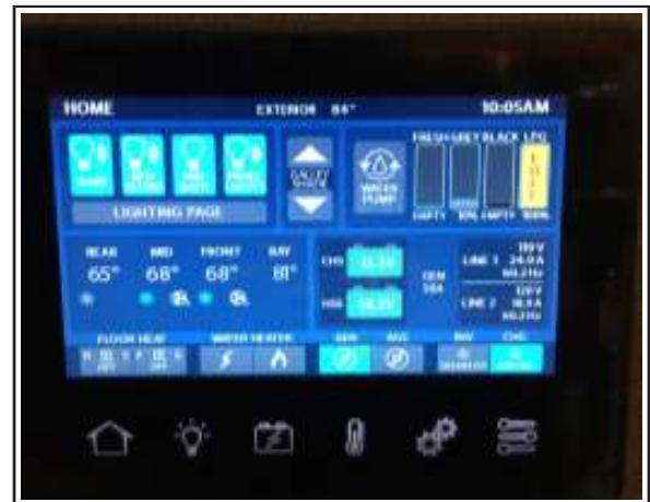
Figure 3-2: Home screen for the Spyder Controls System
