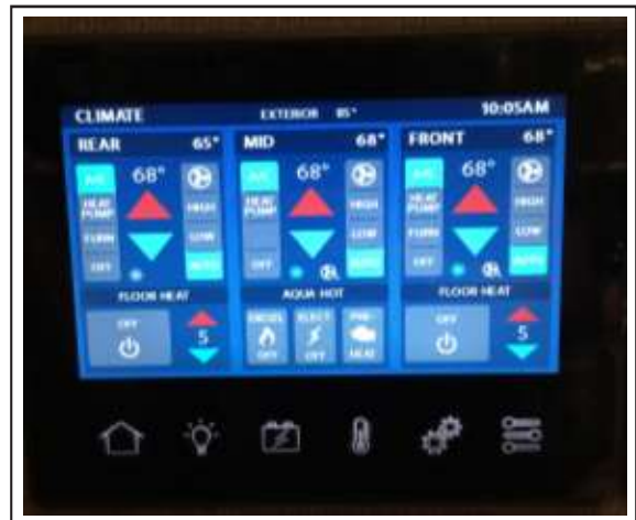
Figure 4-3 Thermostat on Spyder Control System
