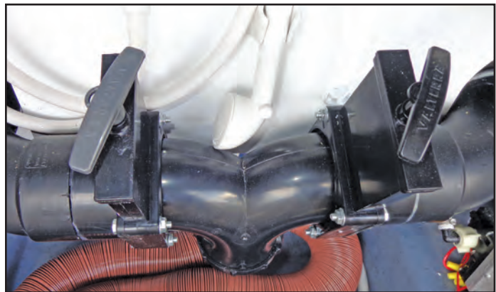
Figure 14-10: Sanitation coupling, valve and hose
