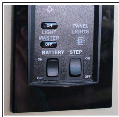
Figure 10-7: 12 VDC disconnect switch
