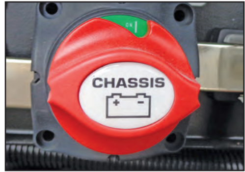
Figure 10-6: Engine battery disconnect panel switch
