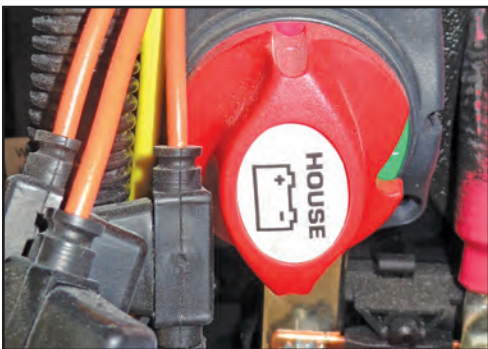
Figure 10-5: House battery disconnect panel switch
