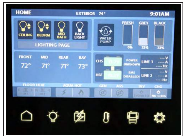
Figure 3-2: Home screen for the Spyder Controls System
