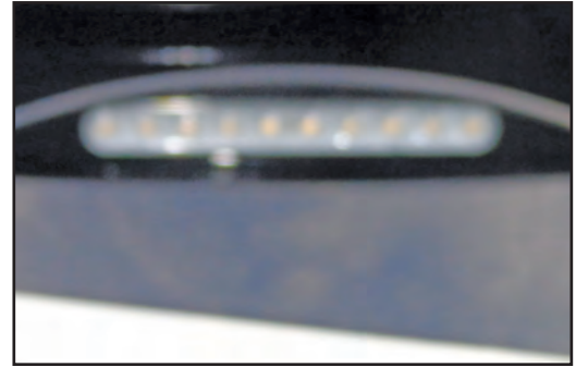
Figure 12-3: Exterior security light
