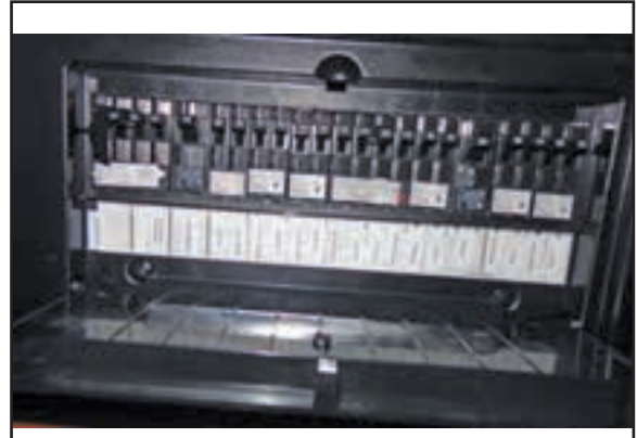
Figure 9-2: Circuit breaker box
