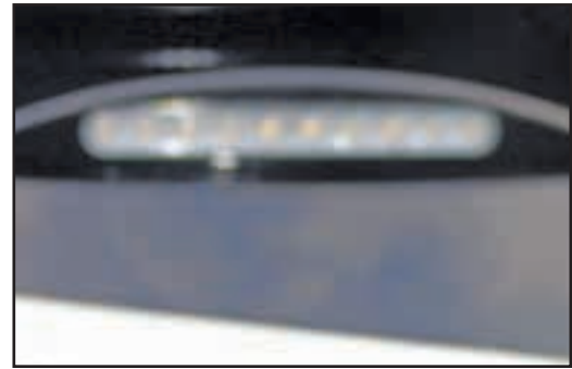
Figure 11-3: Exterior security light
