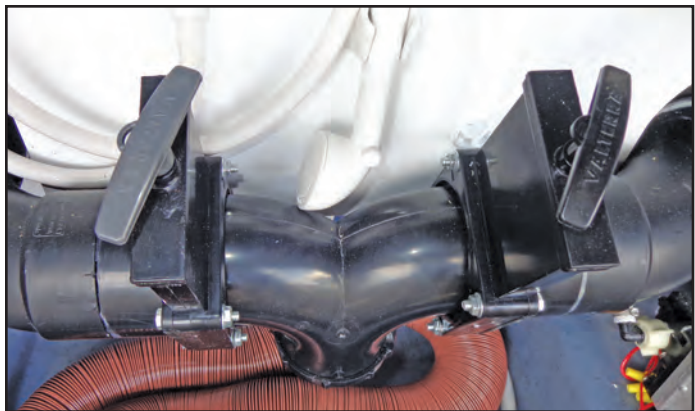
Figure 13-10: Sanitation coupling, valve and hose
