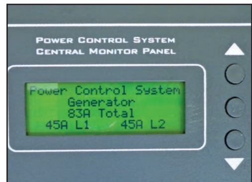
Figure 9-15: Energy management system
