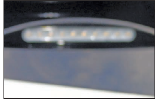
Figure 11-3: Exterior security light
