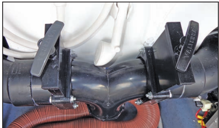
Figure 13-10: Sanitation coupling, valve and hose
