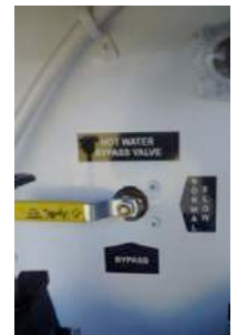
Figure 11-9. Water Heater Bypass System
