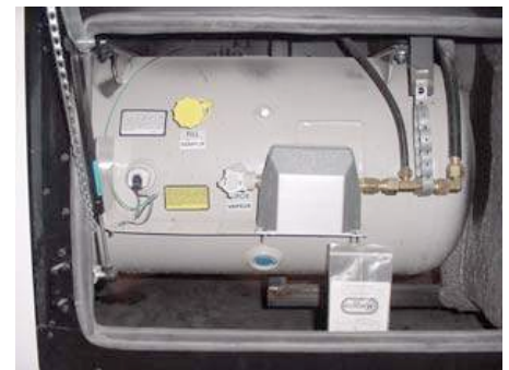
Figure 3-4. Liquid Propane Tank
