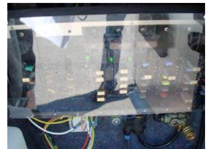
Figure 7-15. Fuse Blocks in exterior compartment on driver’s side
