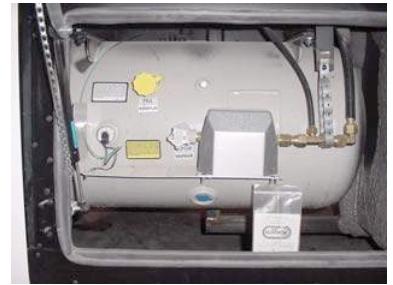
Figure 2-5. Liquid Propane Tank
