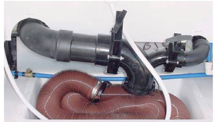
Figure 11-11. Sanitation Coupling, Valve, and Hose
