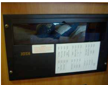
Figure 7-1. Circuit Breaker Box
