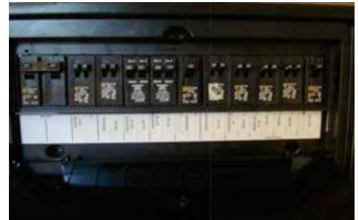
Figure 7-11. Energy Management System
