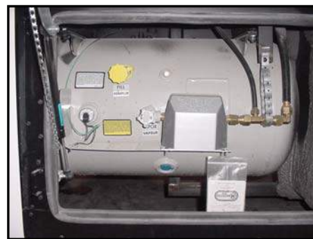
Figure 2-3. Liquid Propane Tank
