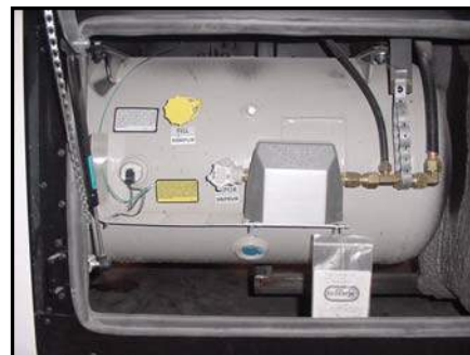
Figure 2-5. Liquid Propane Tank
