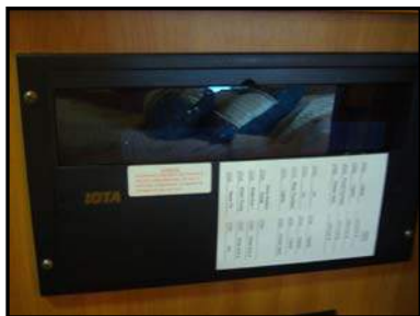
Figure 7-1. Circuit Breaker Box
