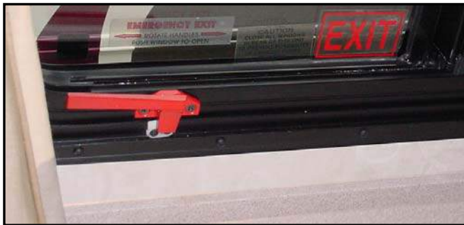
Figure 12-2. Bedroom Emergency Exit Window
