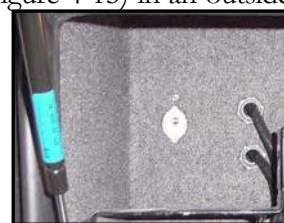
Figure 4-15. Cable & Telephone Jack
