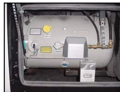
Figure 3-4. Liquid Propane Tank
