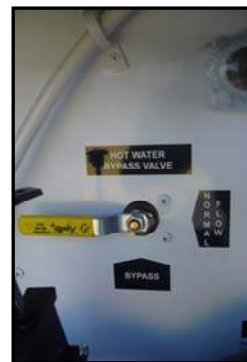
Figure 11-9. Water Heater Bypass System
