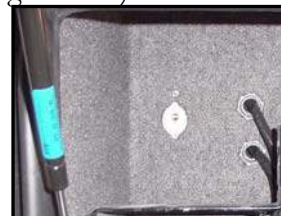
Figure 4-15. Cable & Telephone Jack
