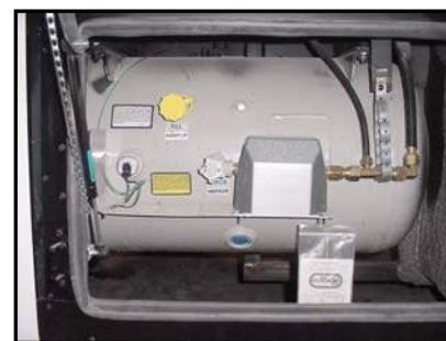
Figure 3-4. Liquid Propane Tank
