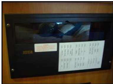
Figure 7-1. Circuit Breaker Box
