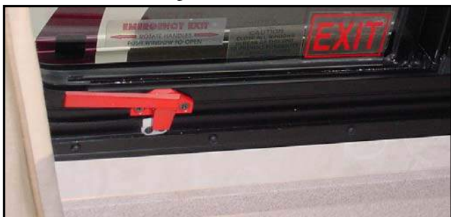
Figure 13-2. Bedroom Emergency Exit Window
