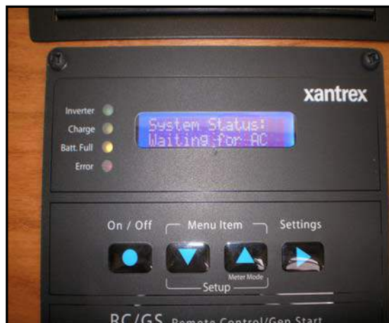
Figure 7-12. Inverter Control Panel
