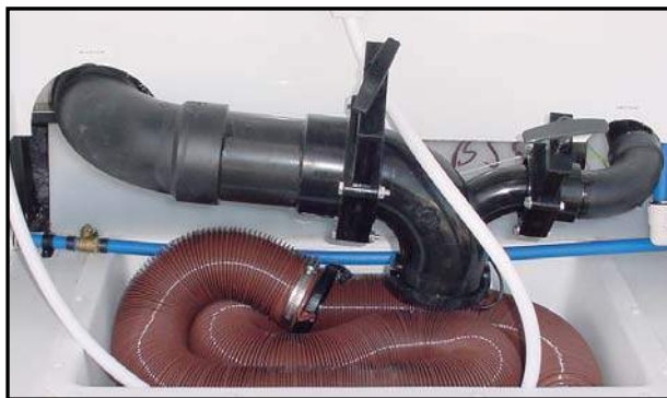
Figure 11-11. Sanitation Coupling, Valve, and Hose
