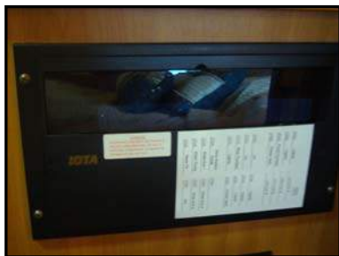
Figure 7-1. Circuit Breaker Box
