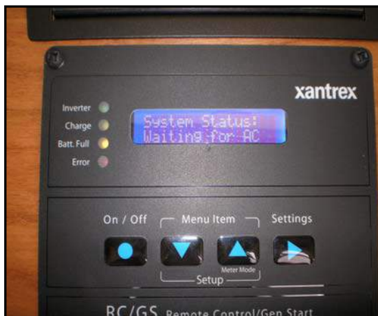
Figure 7-13. Inverter Control Panel
