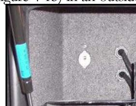
Figure 4-15. Cable & Telephone Jack
