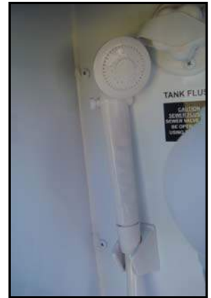
Figure 11-12. Exterior Shower and Exterior Light
