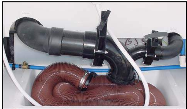
Figure 11-11. Sanitation Coupling, Valve, and Hose
