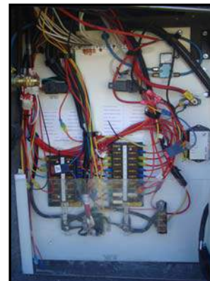
Figure 7-17. Fuse Blocks in exterior compartment on driver's side
