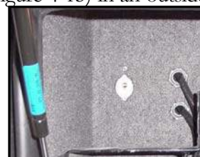
Figure 4-15. Cable & Telephone Jack
