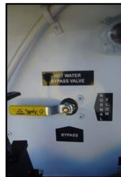
Figure 11-9. Water Heater Bypass System
