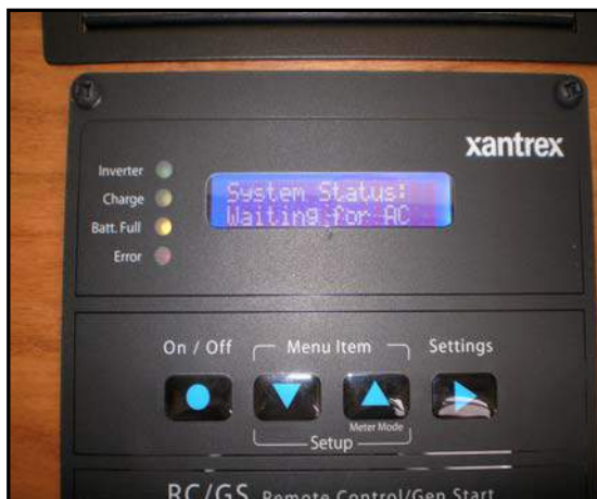
Figure 7-13. Inverter Control Panel
