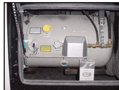
Figure 3-4. Liquid Propane Tank
