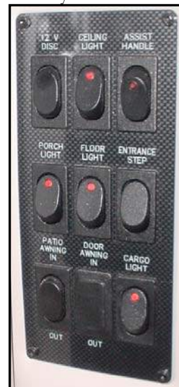
Figure 7-8. 12 VDC Disconnect Switch
