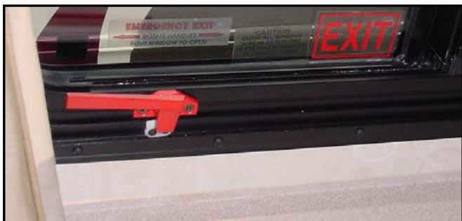
Figure 13-2. Bedroom Emergency Exit Window
