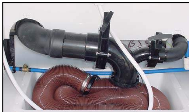
Figure 11-11. Sanitation Coupling, Valve, and Hose
