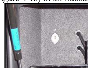
Figure 4-15. Cable & Telephone Jack
