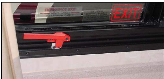
Figure 13-2. Bedroom Emergency Exit Window
