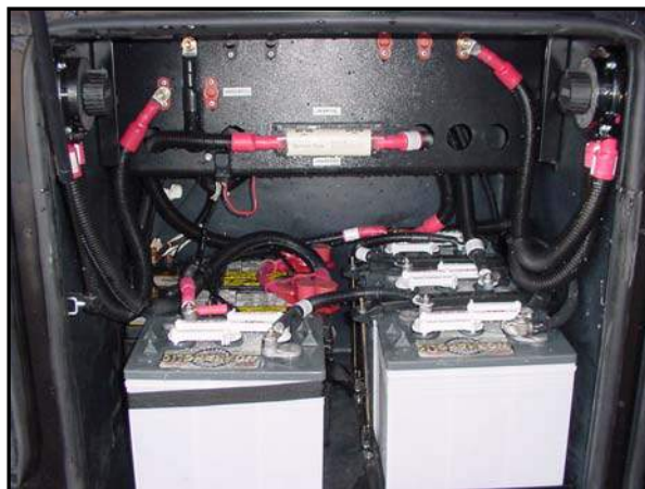
Figure 7-5. 12 VDC Battery System
