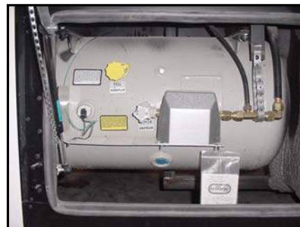
Figure 2-5. Liquid Propane Tank
