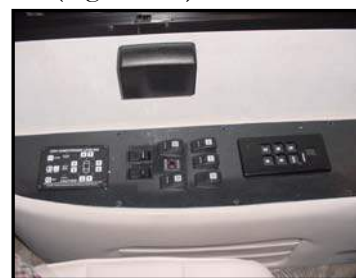
Figure 7-4. Driver's Side Console
