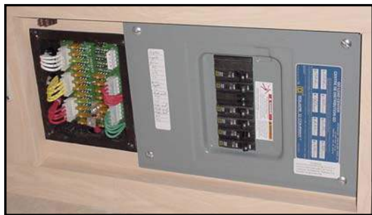
Figure 7-1. Circuit Breaker Box
