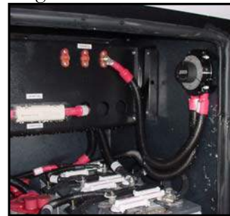
Figure 7-7. House Battery Disconnect Switch (right side)
