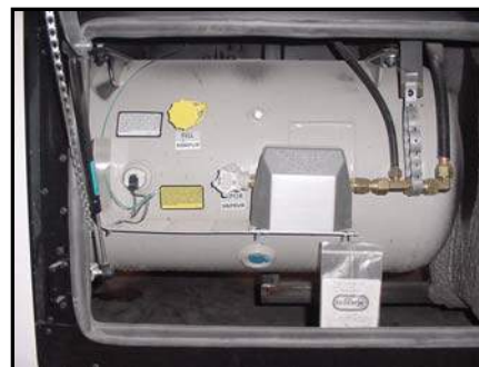
Figure 2-4. Liquid Propane Tank
