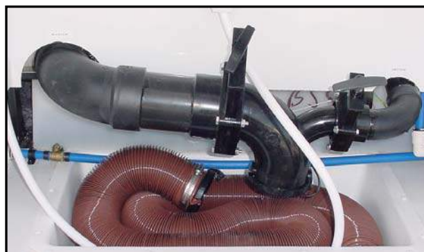
Figure 11-11. Sanitation Coupling, Valve, and Hose
