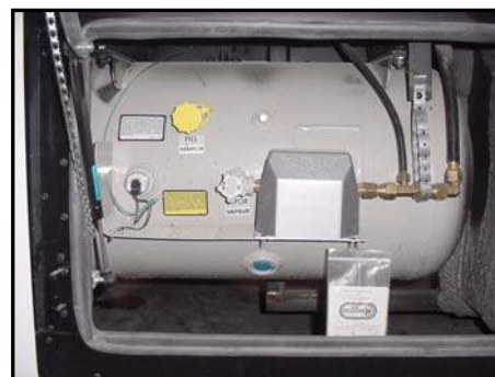
Figure 2-2. Liquid Propane Tank
