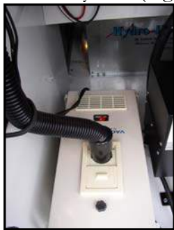
Figure 14-12. Vacuum Cleaner System
