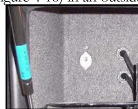
Figure 4-16. Cable & Telephone Jack
