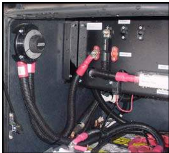
Figure 7-6. Engine Battery Disconnect Switch (left side)
