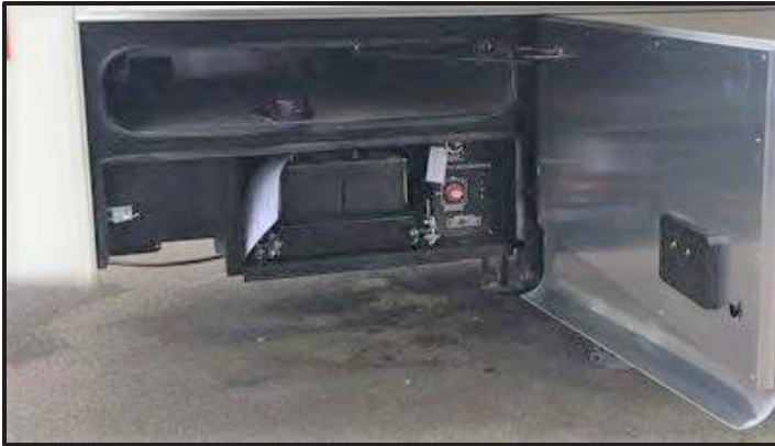
Figure 9-12: House Battery Disconnect Switch
