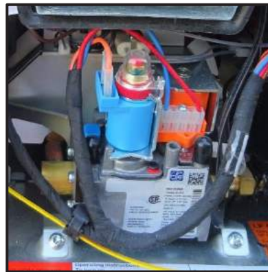
Figure 5-10: Water Heater Relief Valve
