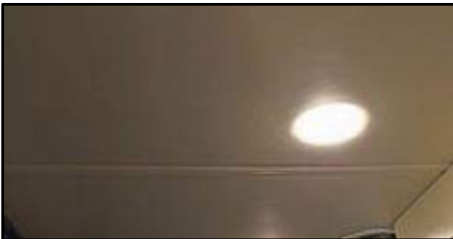
Figure 12-3: Typical Ceiling in the Allegro
