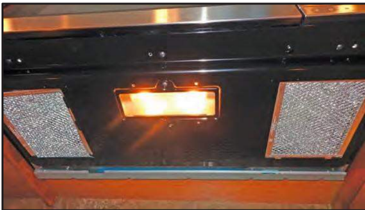
Figure 5-5: Air Filtration Fan
