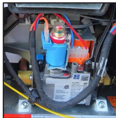
Figure 5-10: Water Heater Relief Valve
