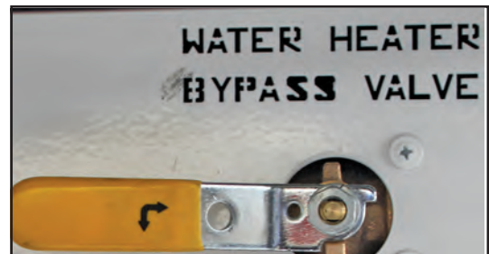
Figure 13-8: Water Heater bypass system
