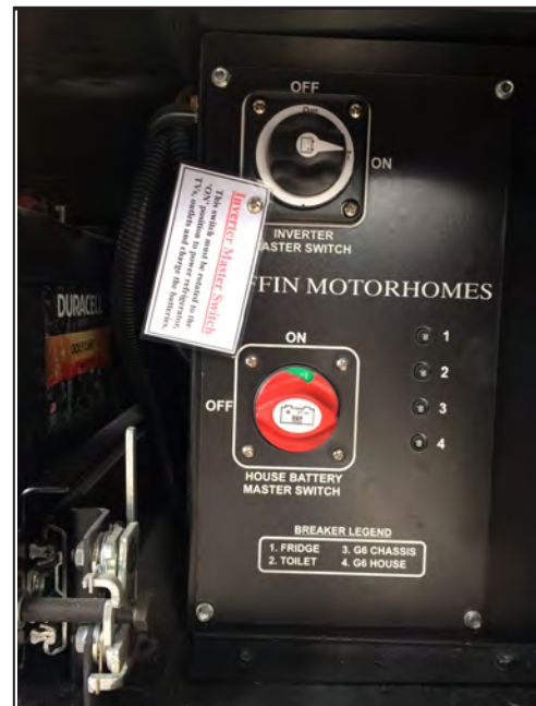
Figure 9-13: Engine battery disconnect switch
