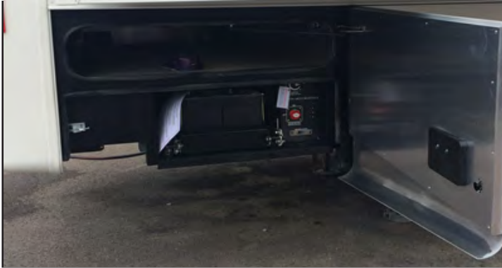
Figure 9-12: House battery disconnect switch
