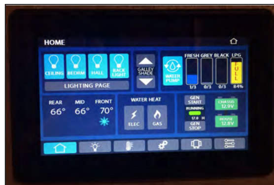
Figure 9-15: Spyder Controls Multiplexing System
