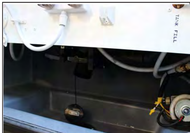
Figure 13-10: Sanitation coupling, valve and hose
