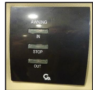
Figure 13-3: Patio Awning Control Switch
