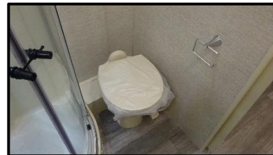
Figure 12-10: Rear Macerator Toilet
