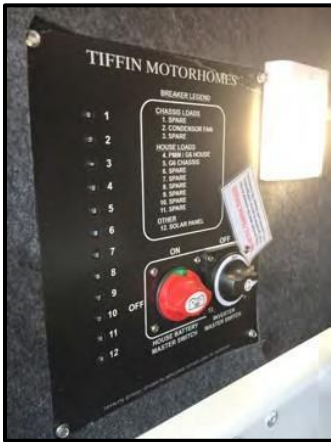
Figure 9-13: House Battery Disconnect Panel
