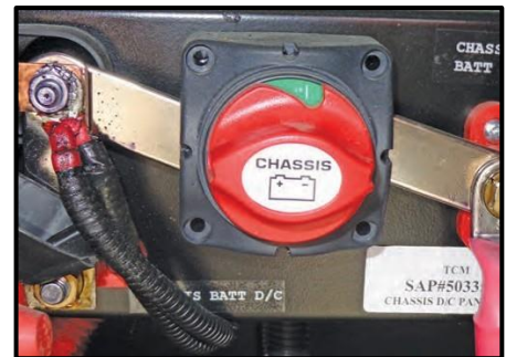
Figure 9-14: Engine Battery Disconnect Switch. Front Wall of Battery Camp
