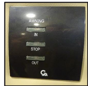
Figure 13-3: Patio Awning Control Switch
