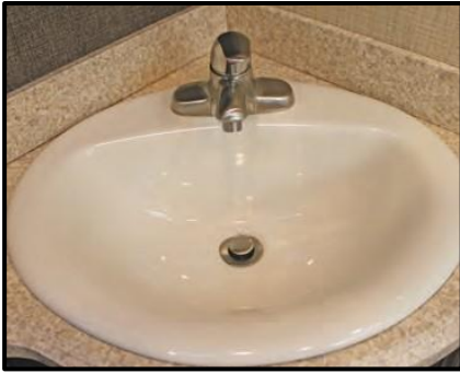
Figure 13-3: Bathroom Sink and Faucet
