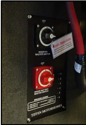
Figure 9-15: House Battery Disconnect Panel
