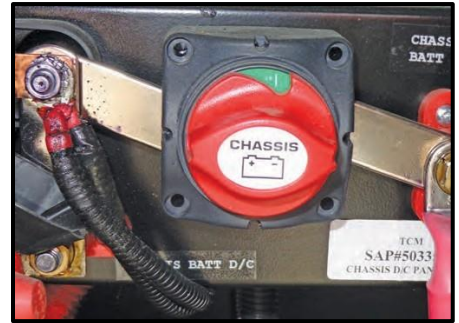
Figure 9-16: Engine Battery Disconnect Switch
