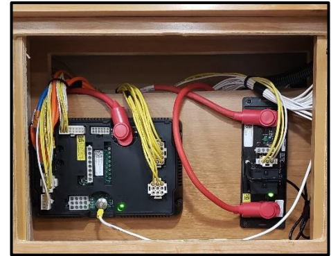
Figure 9-3: Multiplex System Switch Panel
