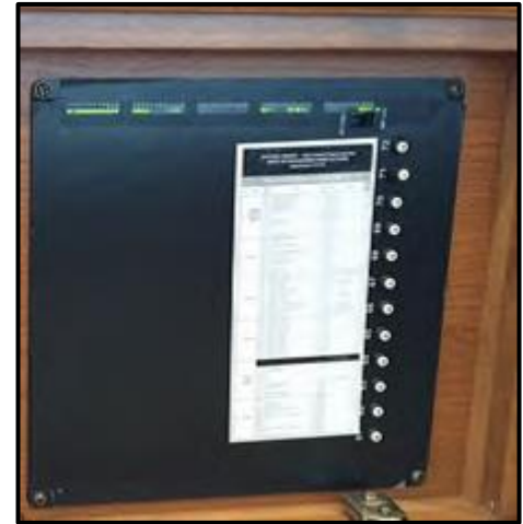
Figure 9-3: Multiplex System Switch Panel
