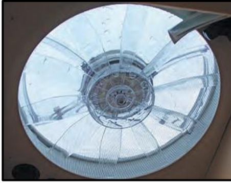
Figure 14-3: Overhead Vent Fan
