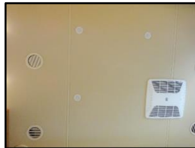
Figure 3-3: Supply Vents and A/C Unit
