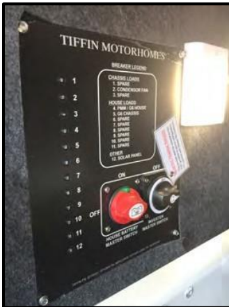
Figure 9-15: House Battery Disconnect Panel
