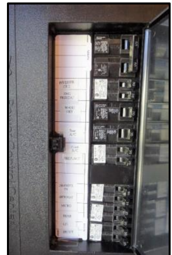
Figure 9-4: Circuit Breaker Boxes
