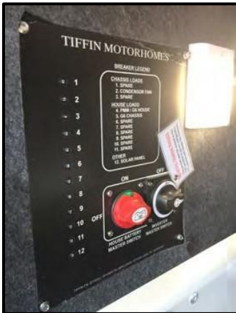
Figure 9-15: House Battery Disconnect Panel
