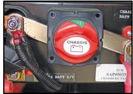
Figure 9-16: Engine Battery Disconnect Switch
