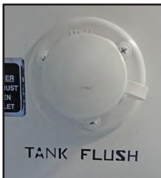
Figure 13-12: Tank Flush Connection
