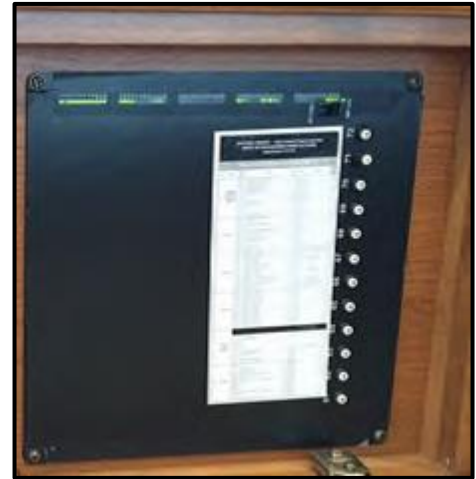
Figure 9-3: Multiplex System Switch Panel
