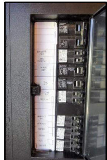
Figure 9-4: Circuit Breaker Boxes
